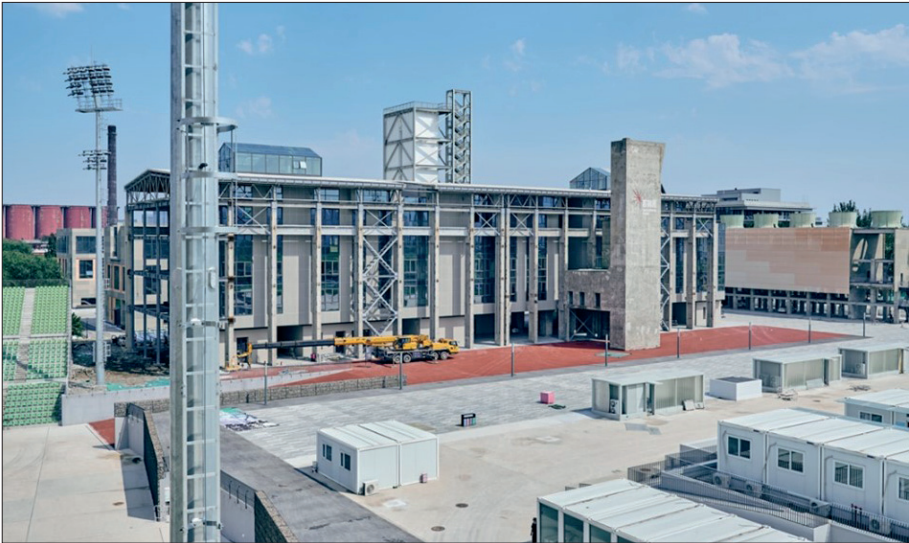
Fig. 9. Reconstruction of the North District of the Oxygen Factory (Photo ©Lu Bei)
