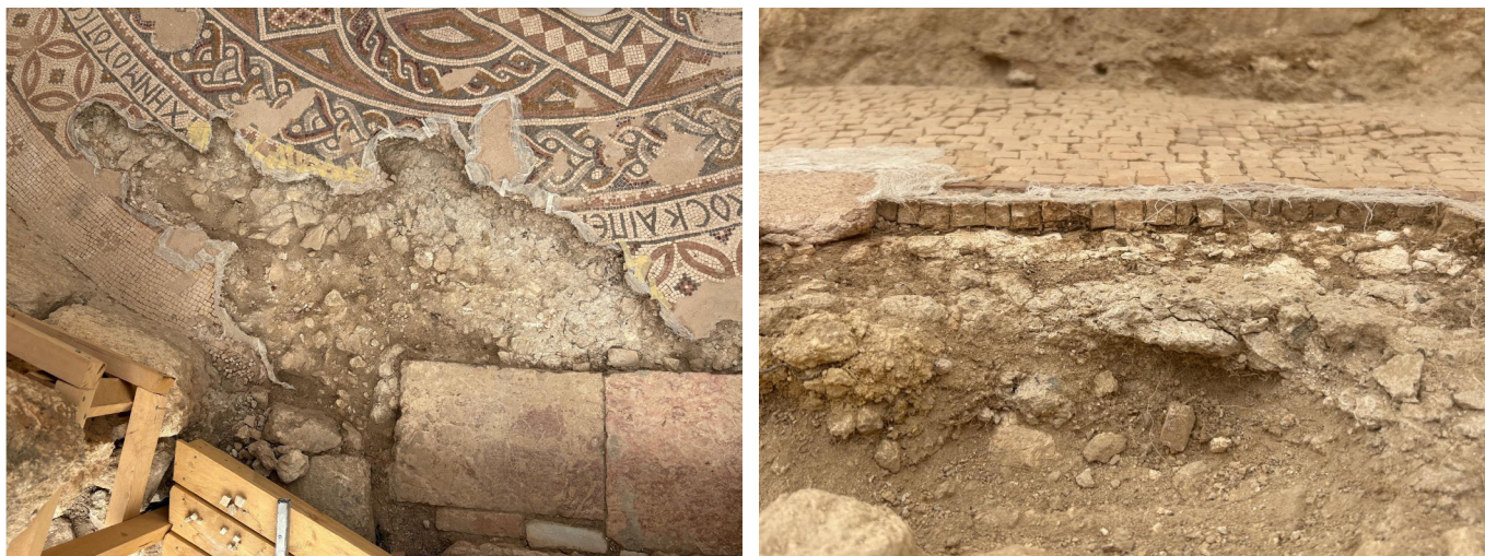
from left, Fig. 5a view of the largest gap located at the entrance to the room.
